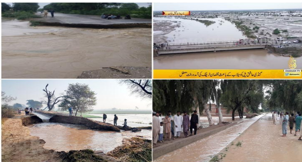
Figure 3: Structural damage of flood to roads, bridges, and canal breaches in Dera Ismail Khan
